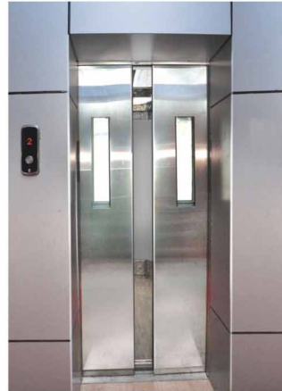
S.S. Center Opening Auto Door
